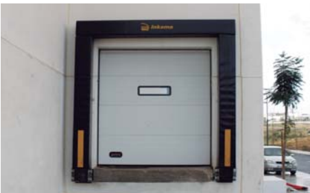
Cold store dock shelter
