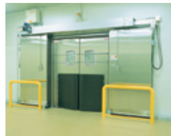
冷蔵庫 Refrigerating room
