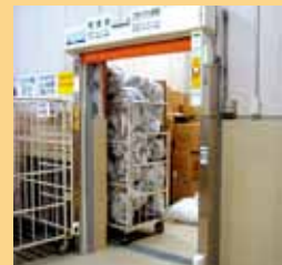
▲Installation example (Supermarket)
